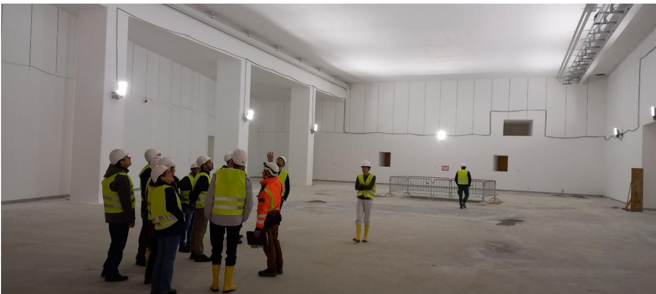
Figure 1: picture of the visit of FAIR. Participants of the THRILL End-User Workshop visit the FAIR construction site in Darmstadt, Germany. [Picture: B. Zielbauer]
